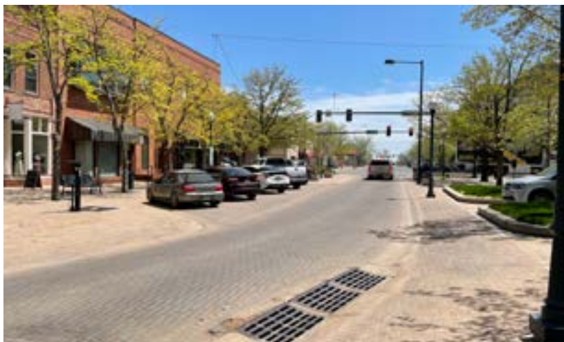
Image of unit pavers in vehicular area, concrete flow line with drain inlets, and streetscape along 8th Street
