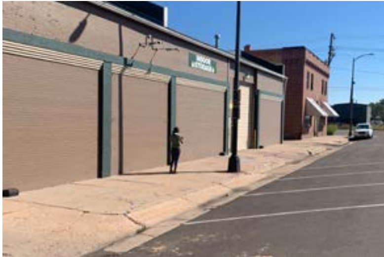
Image of a blank facade and dilapidated sidewalk east of 8th Avenue
