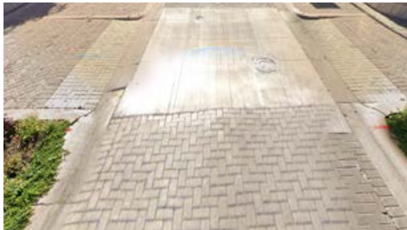
Image of existing unit pavers and colored concrete area on 8th Street needing repair and maintenance
